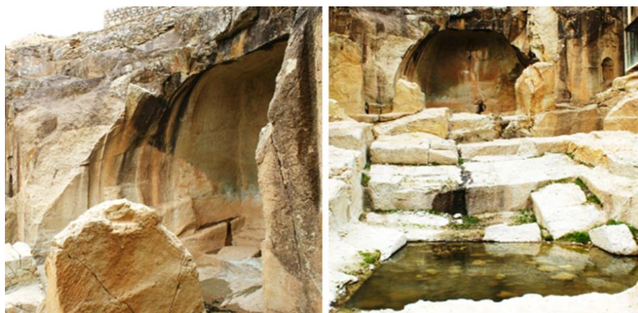
Fig. 5. Left: Missing parts of the central niche caused by geologic erosions; Right: Square pond in the central axis of the complex filled by the runoff from the central niche.
